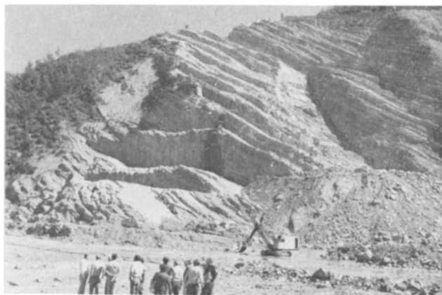
Figure 9. – Ridracoli dam – Excavations for the right abutment; note the anchor heads at the exposed flysch beds.
